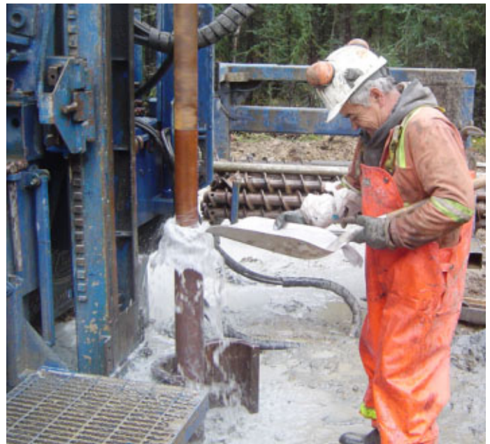
Bedrock drilling is necessary to help determine engineering design for Mayo B.
